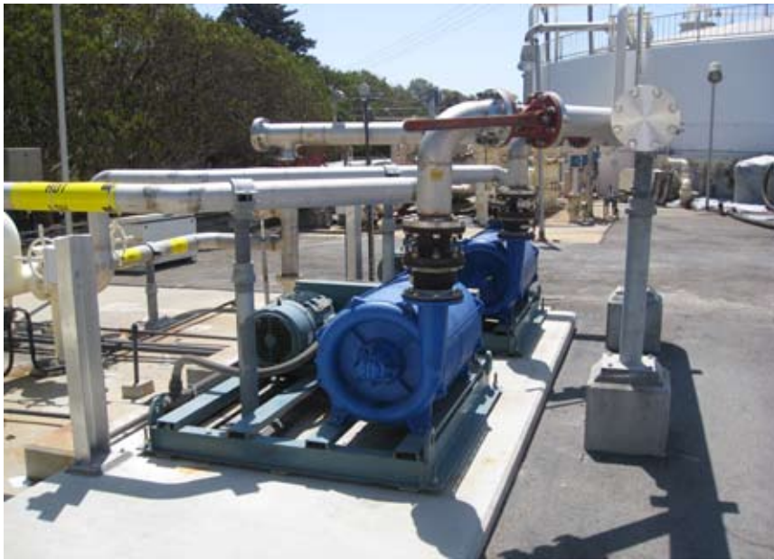
Biogas/Natural Gas Compressors and Equipment Photo
