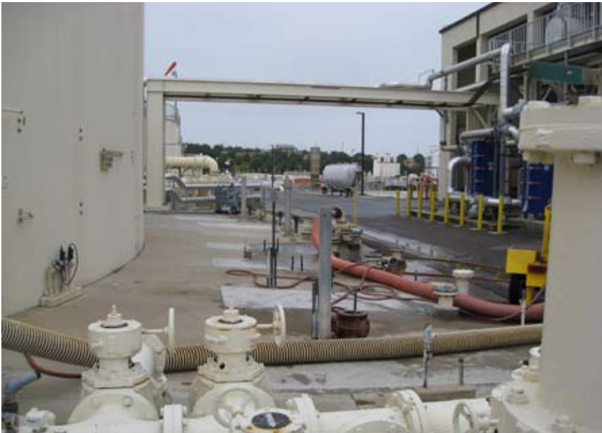
Digesters and Cogeneration Engines Building Photo
