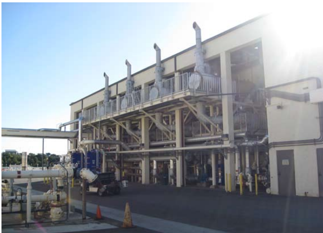
The 5th engine would be added in the existing open bay at the south end of the engine building, pictured here
