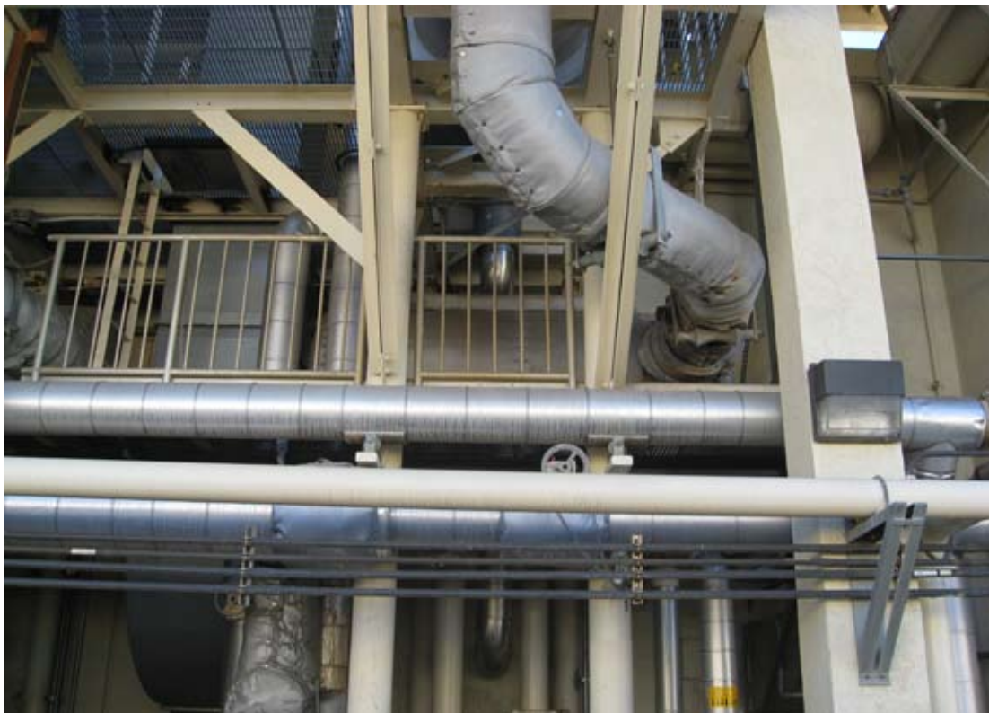
The catalyst would be installed in the existing catalyst housing, pictured here.
