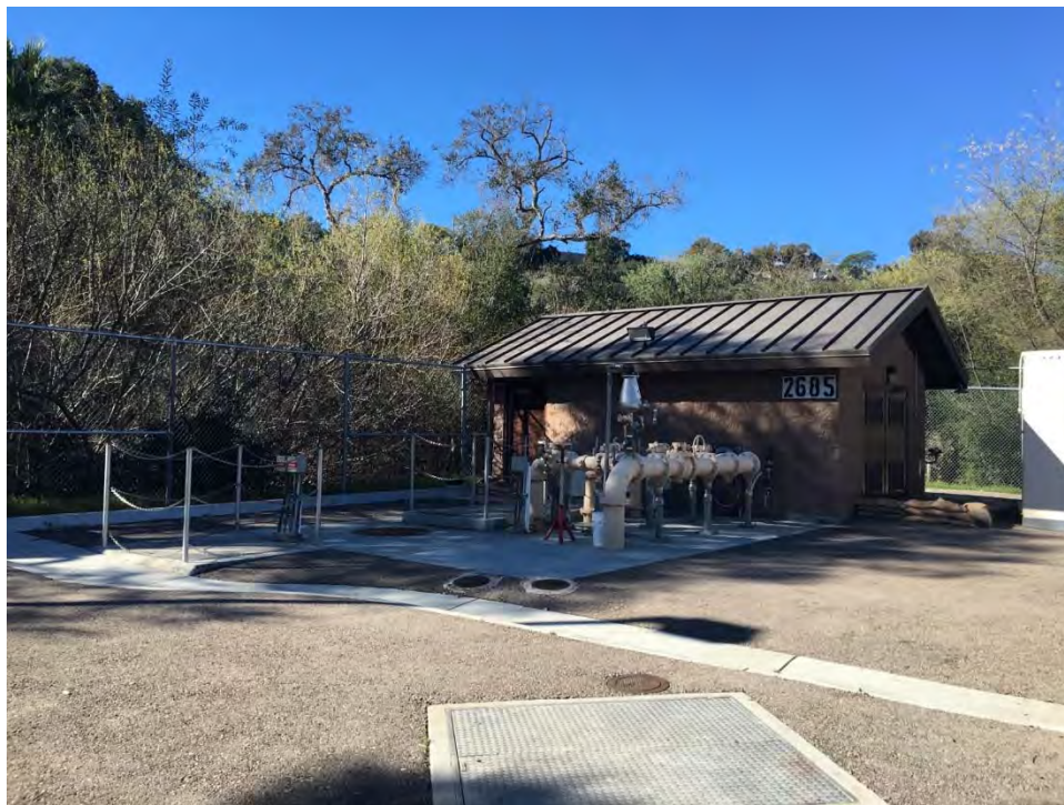
Raceway Basin Pump Station
